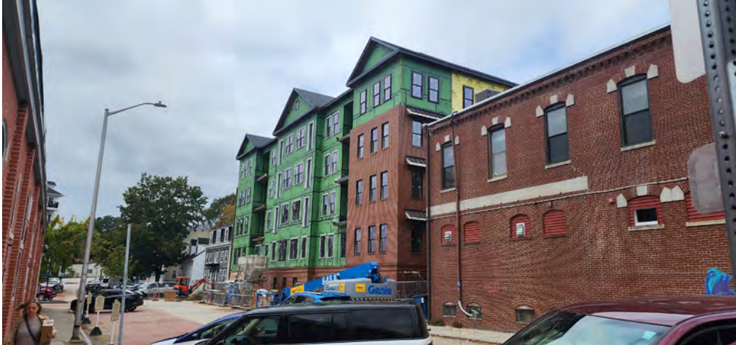
Old Strafford Courthouse during redevelopment construction. Photo from the City of Dover.
